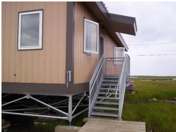
A multipoint structural foundation used to maintain stability of buildings on thawing permafrost, Newtok, Alaska. Credit: Alaska Department of Military and Veterans' Affairs
